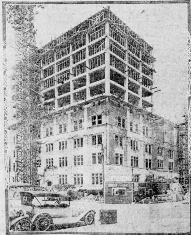
The exterior of the new 12-story Y. M. C. A. building, Ninth street and Mary place, which is being developed in pink brick and white limestone in modified Gothic style, has been completed up to the sixth story. The plastering has been begun on the first floor, and J. L. Robinson, contractor, promises that the building will be ready for occupancy by January 1, 1919.
