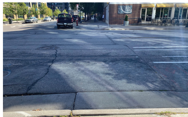
Poor pavement quality on 2nd Street
